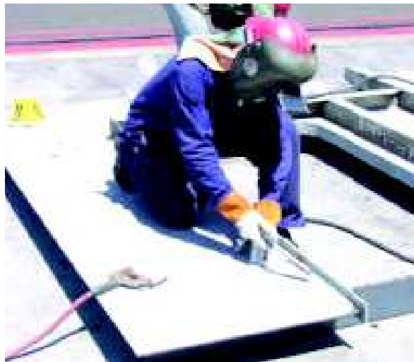
Figure 19 Ground Clamp Not Connected
