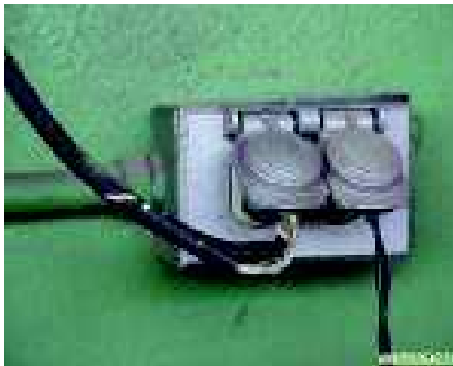
Figure 30 Damaged Insulation and Plug
