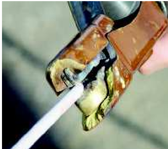
Figure 16 Damaged Electrode (Energized)
