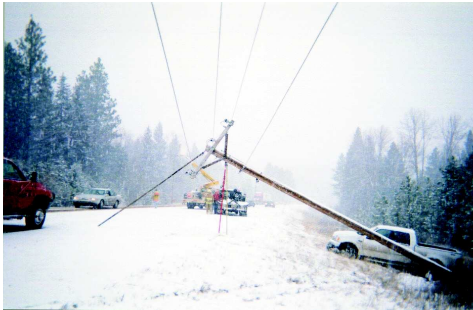
Figure 35 Downed Power Line
